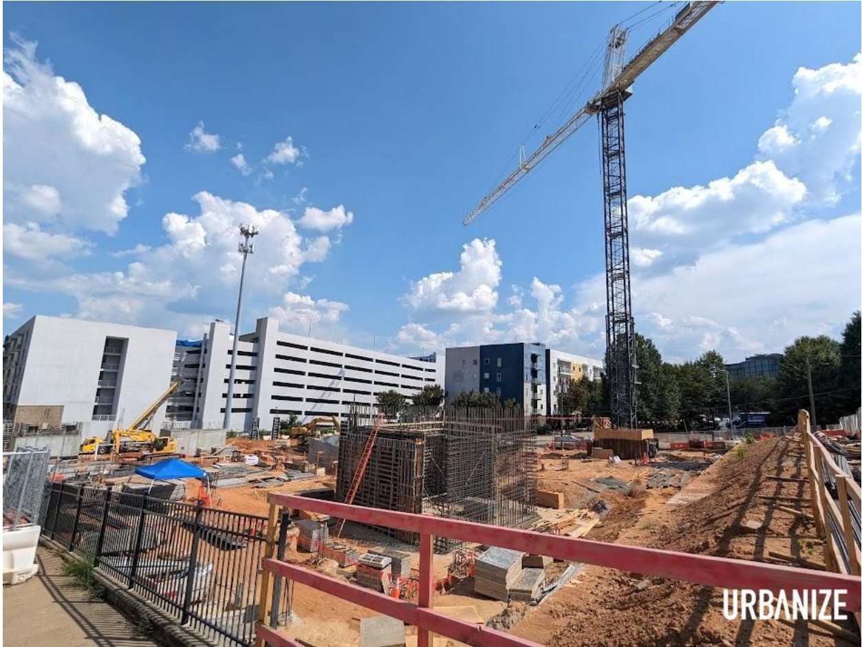
A crane towering over the beginnings of vertical construction at Allen Morris Company's Stella at Star Metals project this past weekend. Josh Green/Urbanize Atlanta
